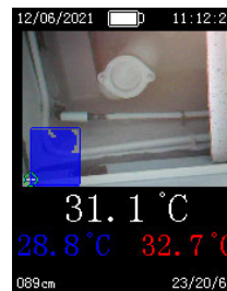
Data Logging, Auto trace and capture water leaks (low temp.) every 60 seconds and stored in micro SD card
