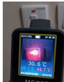
Fault finding of Loose connection inside the switch
