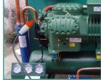
For industrial HVAC air-conditioning
